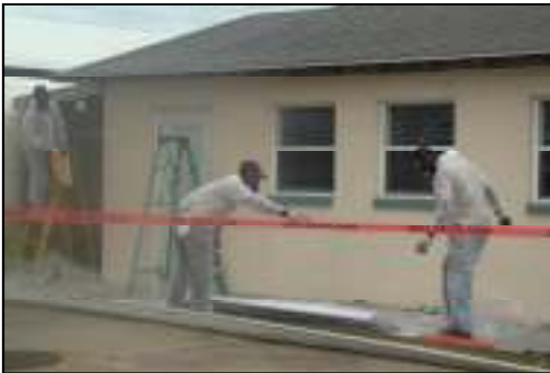
While we eagerly await our official Groundbreaking, preliminary work has begun! Workers, above, remove asbestos from back building prior to its demolition.
